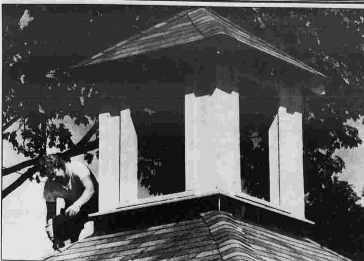
ROOF JOB — Ronald Kenney of South Bolton, an employee of Spear Contractors of Andover, caps the roof on a garage at 271 Plymouth Road, Bolton, on a garage at 271 Plymouth Road, Bolton, on Wednesday.
